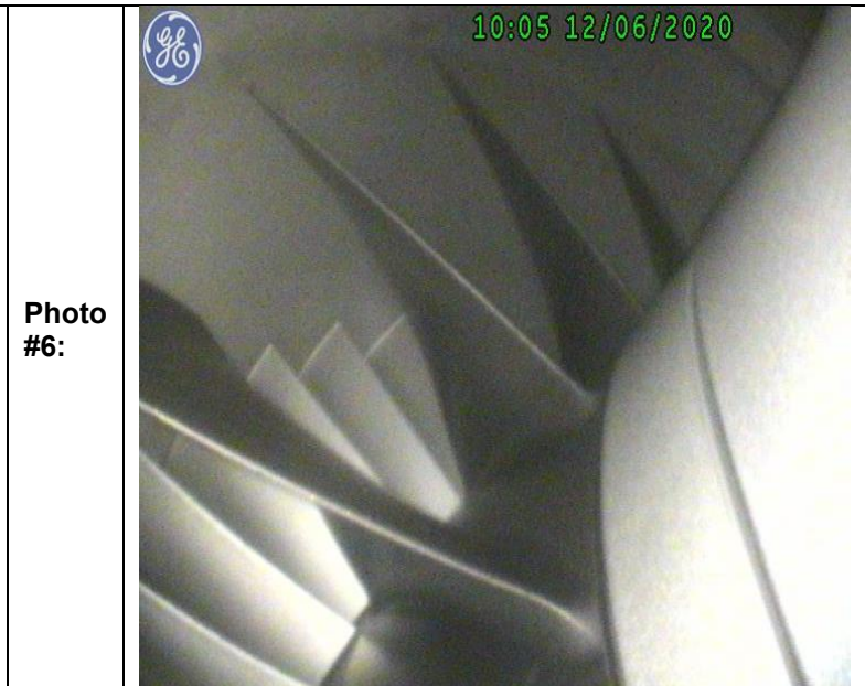
1 st Stage Stator: Acceptable
