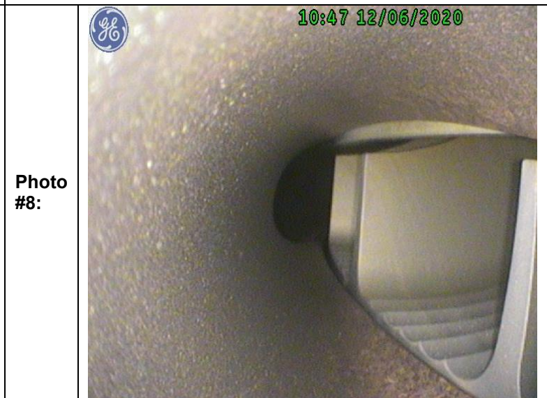
Diffuser block and Centrifugal Compressor outlet: Acceptable
