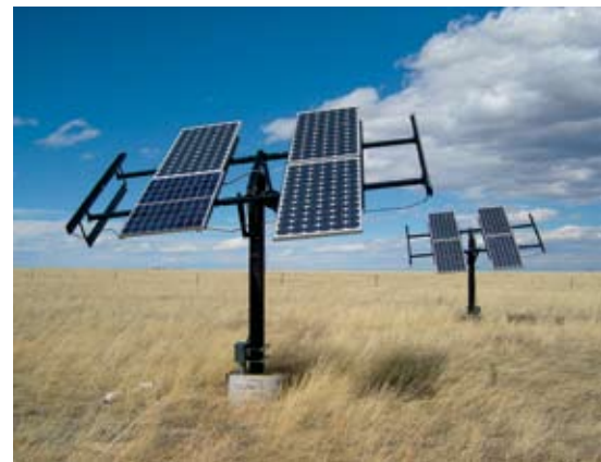
These south-facing photovoltaic (PV) panels produce electricity from sunlight, which is then stored in large batteries for later use. The panels are on motorized bases that track the sun; this is particularly important in the summer, when there is less wind and the sun makes its largest arc across the Wyoming sky
