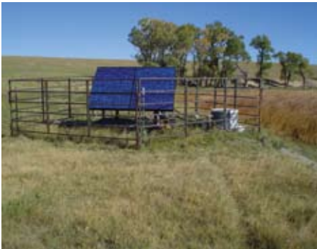
Figure 5. This solar-powered stock water well is drilled only a few feet deep in the middle of an arid basin. It is situated only a few hundred feet away from a perennial stream and taps into sands in the stream’s flood plain, which is saturated with river water. The cottonwoods in the background are a sure indicator of shallow ground water.
