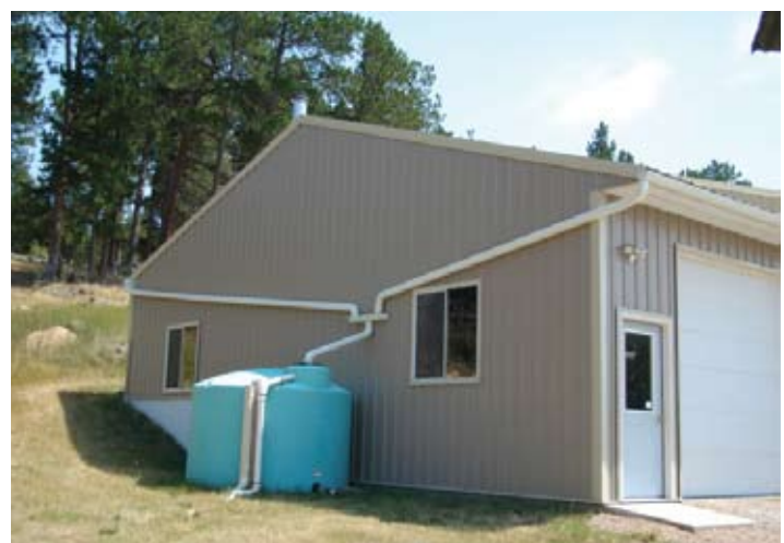
Everard installed a 1,500-gallon storage tank to collect rain from his shop roof. One .90 rain fills the tank.
