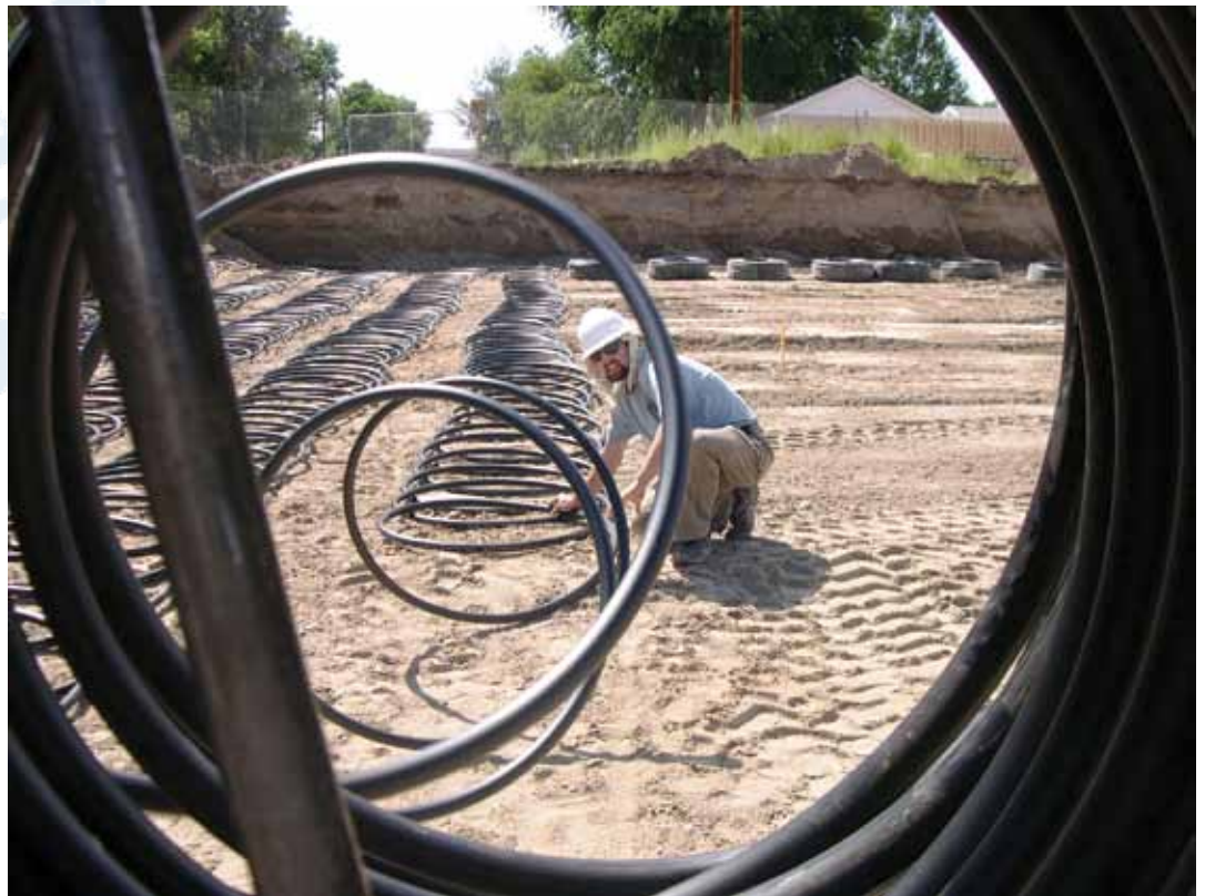
Building a large geoexchange field requires large amounts of space. This is at Greybull Elementary School in Greybull, Wyoming. (Courtesy of Creative Energies)
