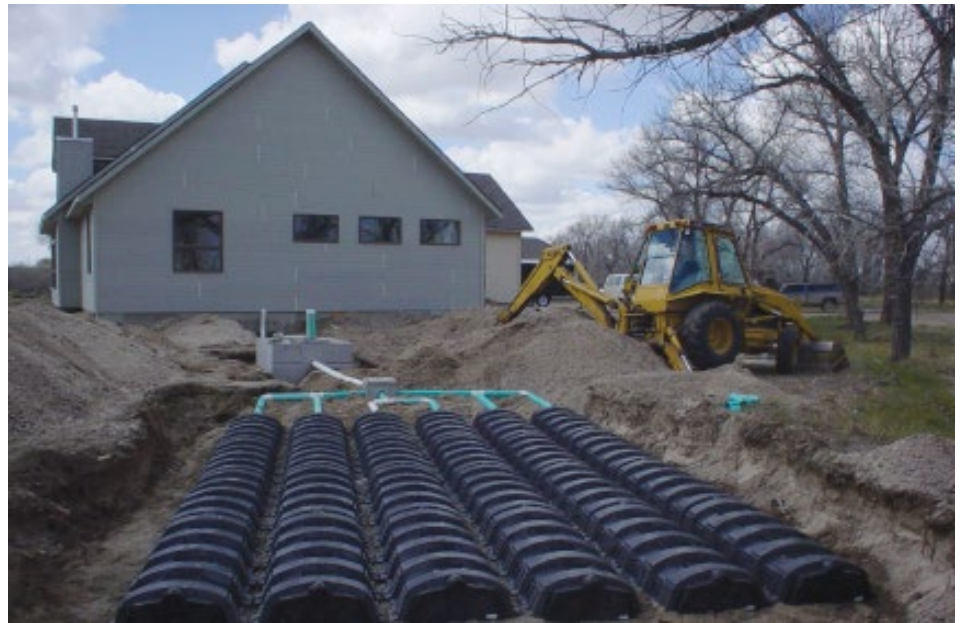
Conventional gravity fed septic system with concrete tank and distribution box. Drainfield is a bed configuration with gravelless chambers.
