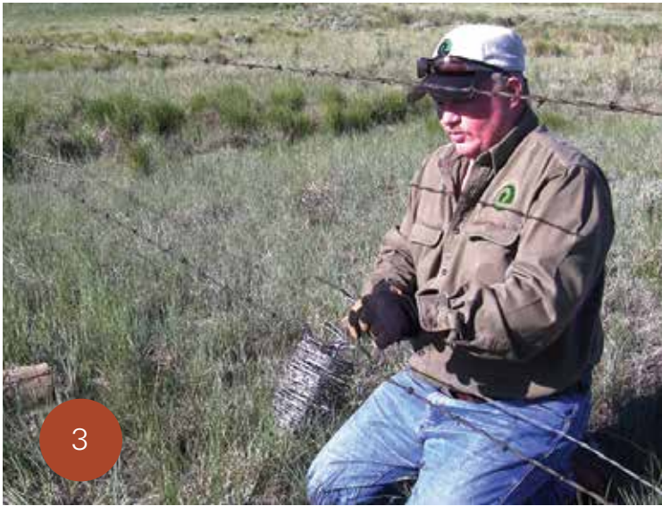
Insert the free end of the roll of barbwire into one of the loops that was created in Photo 2 and create a loop with this piece to attach it to the broken fence loop.
