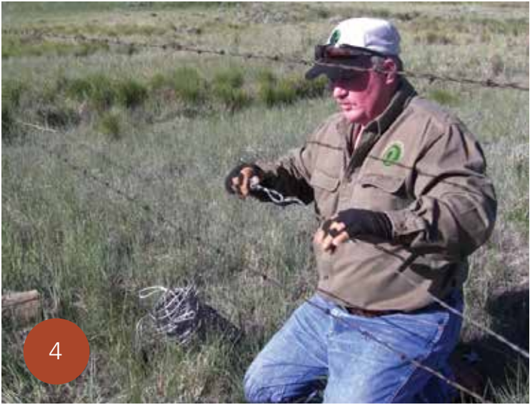
Here is a completed splice of old barbwire attached to the new barbwire.
