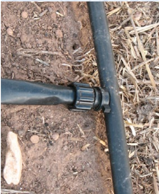
Rows of drip tubing can be attached to a main header leading from the water spigot.
