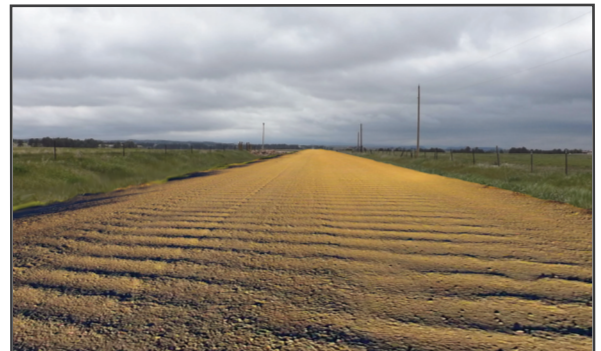
Typical washboard damage on an unpaved road (Source: Jo Michele Sheridan).
