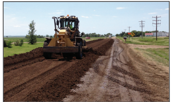
The entire berm must be considered in developing and deploying TTC. (Source: EquipmentWorld).
