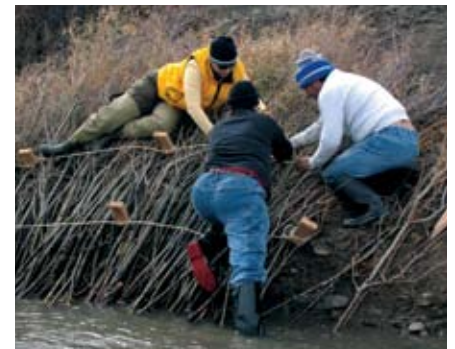
Brush-mattress technique consists of live woody plant material placed into the slope face along trenches excavated along slope contours.
