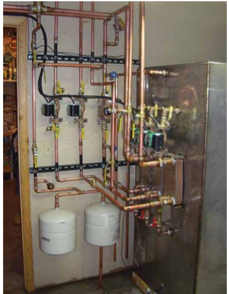
Figure 5 – Non-toxic antifreeze in a closed loop is circulated through a heat exchanger in a backup water heating tank.
