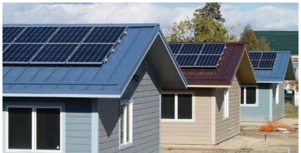
PV and solar thermal installation by Creative Energies of Lander. Photo courtesy Scott Kane.
