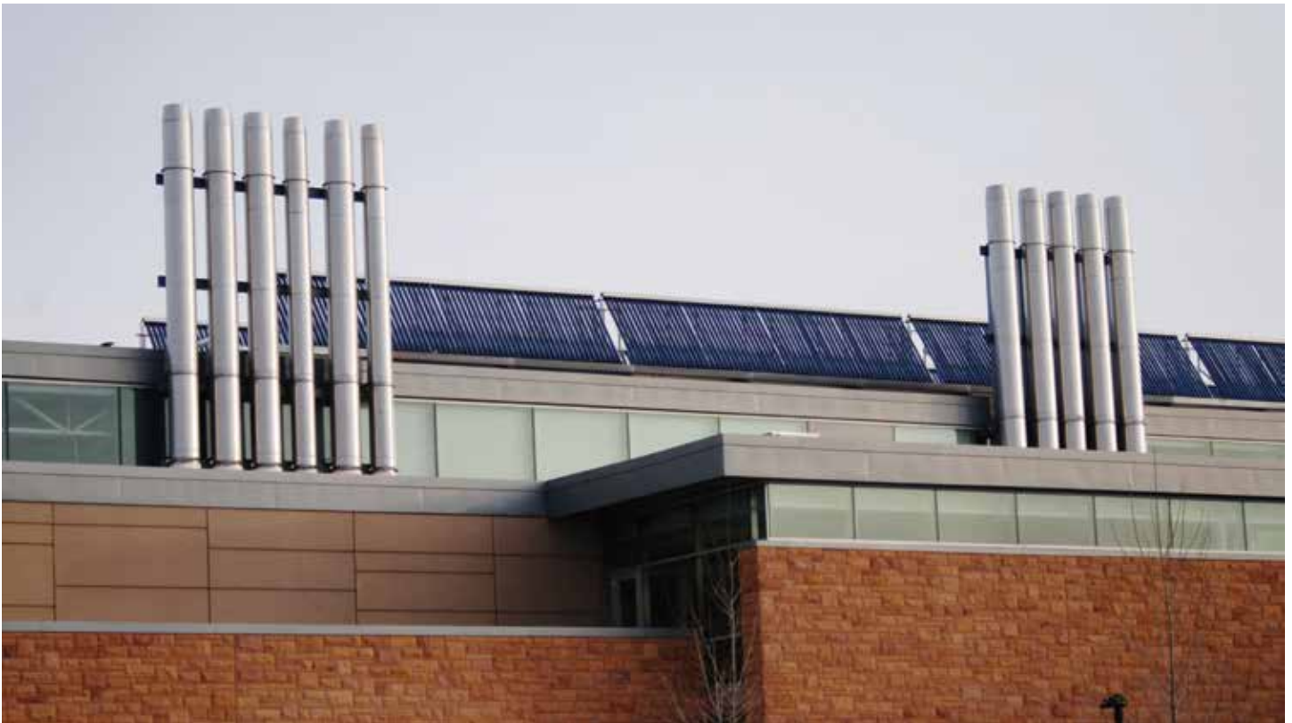
Solar thermal “evacuated tube” heating system on the roof of the UW Visual Arts Building. These active solar systems are an integral part of the aesthetic design and are not perceived as an eye-sore by most.
