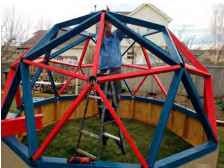
Nearly completed dome frame. Red struts are the shorter "A" struts with 16 degree angles on both ends. Blue struts are the longer "B" struts with 18 degree angles on both ends.
