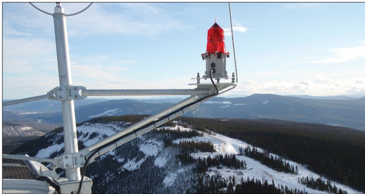
An obstruction lighting unit atop the 144 MW Dokie Wind Farm, located near Chetwynd, British Columbia.
