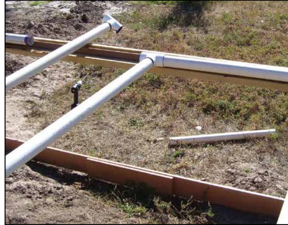
Figure 20. Scab over butt joint of base plate.
