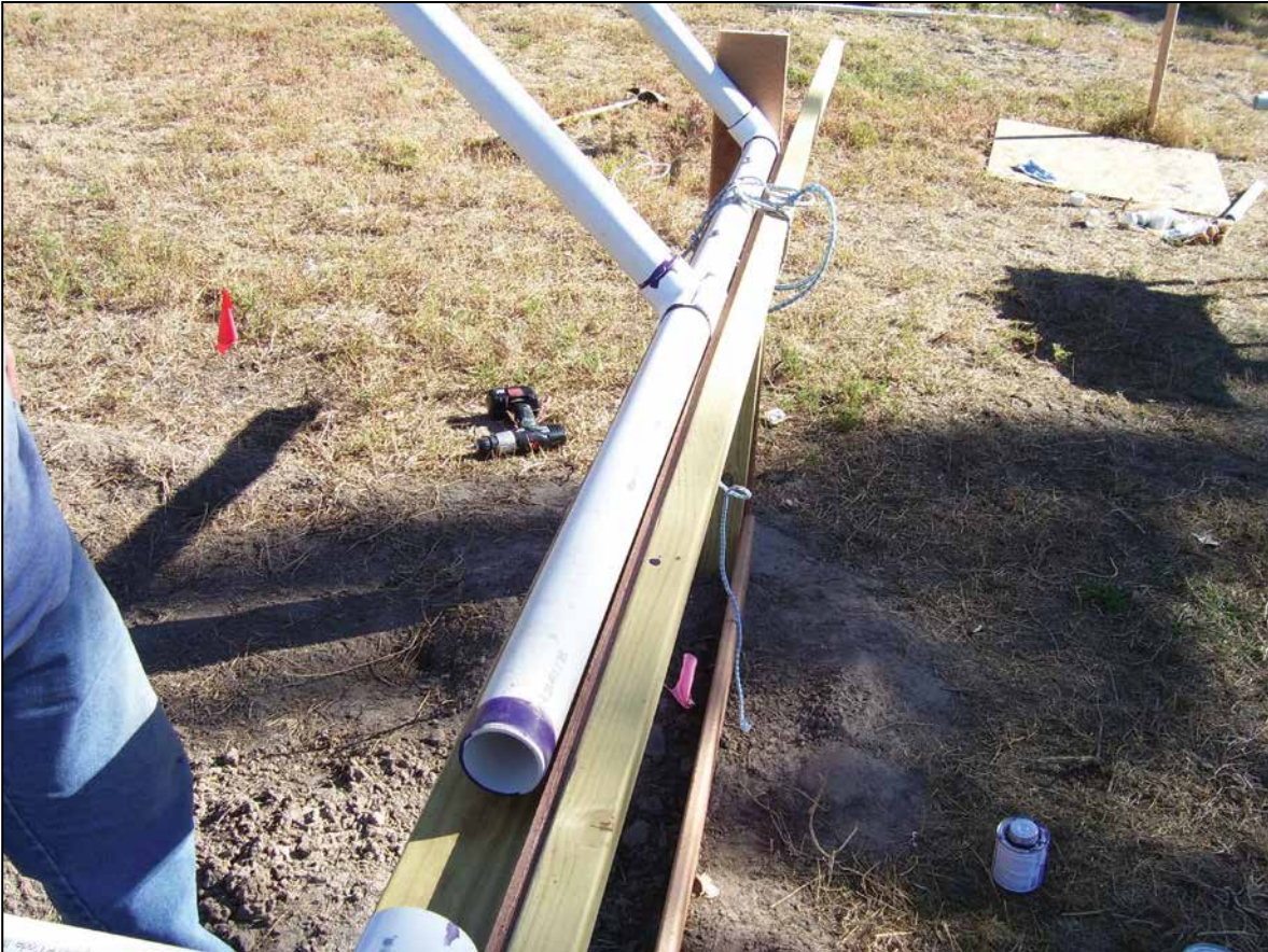
Figure 16. Spacer cleaned/primed and cemented into “T” joint of the first rib assembly.
