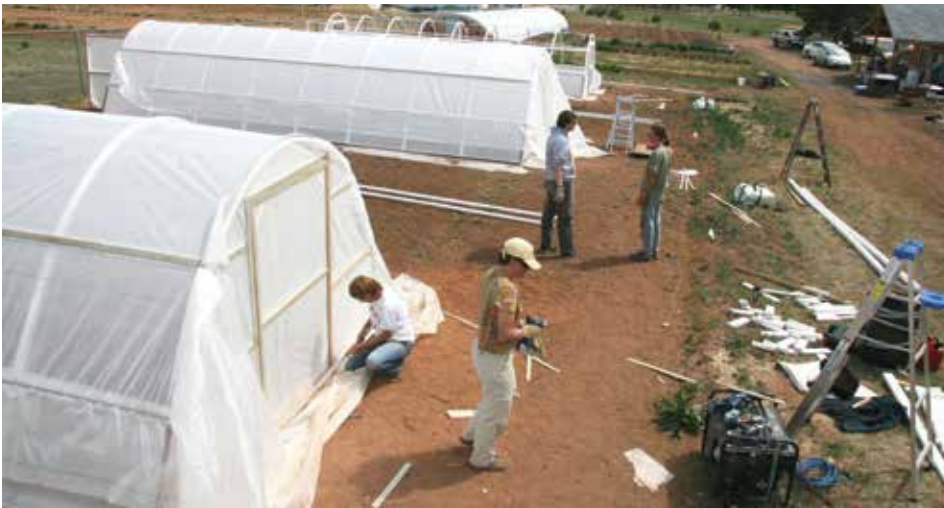
Volunteers built five hoop houses for ACRES at the Laramie Research and Extension Center greenhouse complex.
