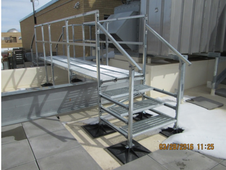
ROOF WALKWAY & STAIR WITH NON-PENETRATING BASES
