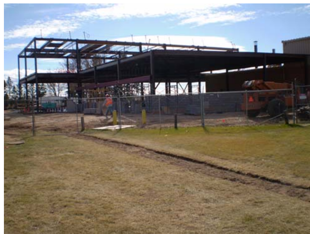
Oct 2009. All of the foundation is poured, structural steel has been erected, and the cinder-block walls are going up.
