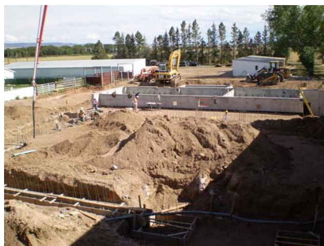
July 2009. The new addition is a big hole in the ground with some foundation poured.
