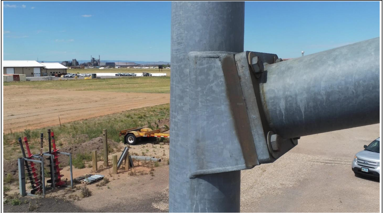
Figure 2 Inspection photo captured by a Parrot Anafi UAV showing general level of detail provided by prosumer level equipment. Assets such as this overhead traffic signal mast can safely and quickly be inspected by utilizing UAS
