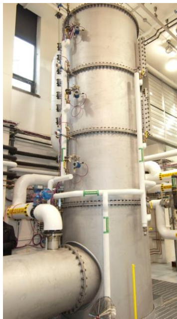
Figure 3. – 1 MWt Oxy-combustion furnace at the Advanced Coal & Energy Research Facility (ACERF)
