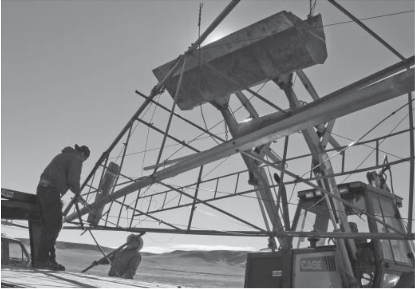
Developing water resources on the Y Cross Ranch has allowed the operation to graze livestock in areas previously not used. Ranch Manager Manny Monserrate, center, helps Lawrence Walters, left, and backhoe operator Paul Schumm of Paul's Well Service & Sons of Cheyenne unload a windmill that will pump water from a recently drilled well in an isolated pasture.
